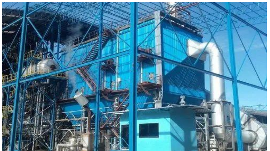
Boiler Electrostatic Precipitator (ESP).
