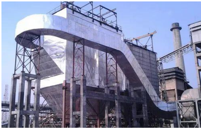
Retrofit Electrostatic Precipitators
